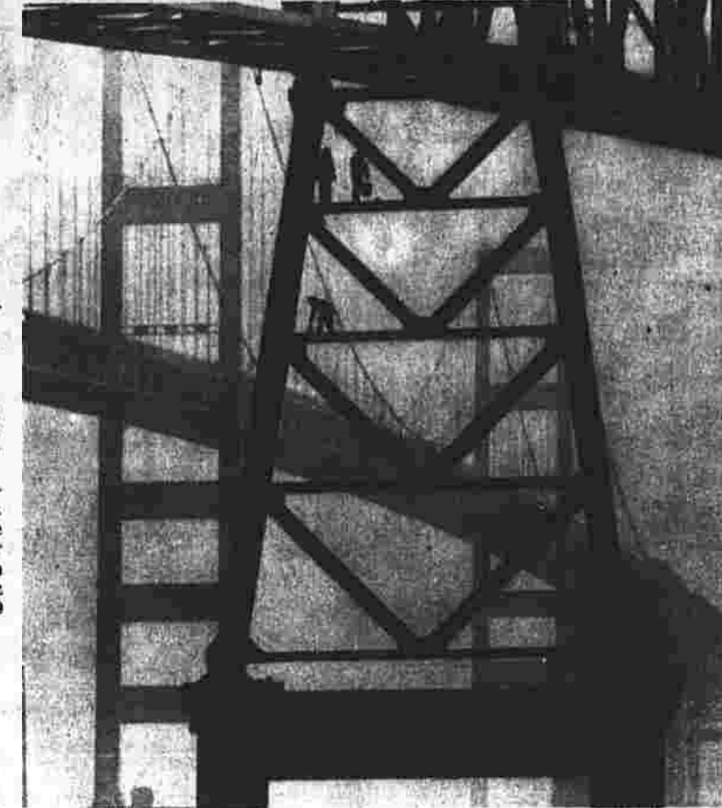
Foggy morning Painters work on a support of the eastbound span of the Chesapeake Bay Bridge while the westbound span looms in the background, partly obscured by early morning fog.
